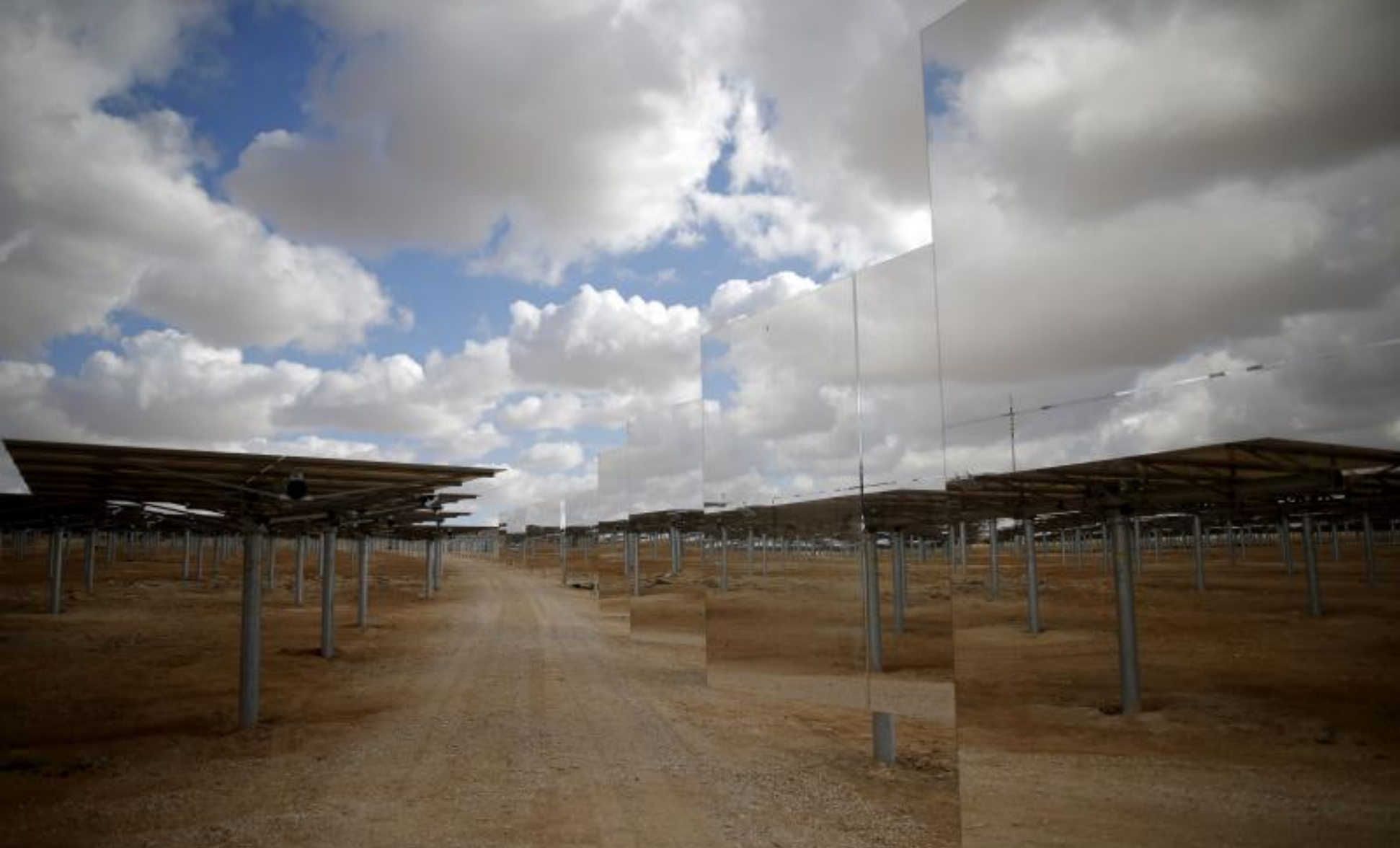
Heliostat mirrors reflect their surroundings in a field at the construction site of a 240 meter (787 feet) solar-power tower in Israel.
